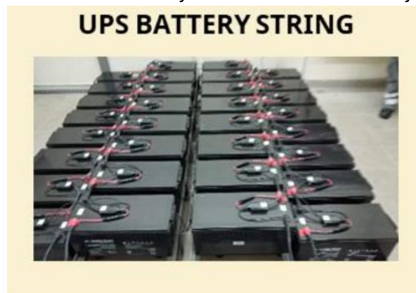
Figure 6: UPS Battery String.
