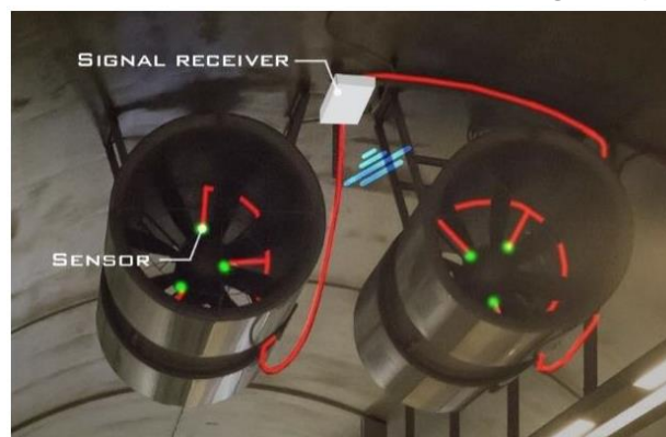
Figure 3: Installed vibration sensors on a jetfan.
