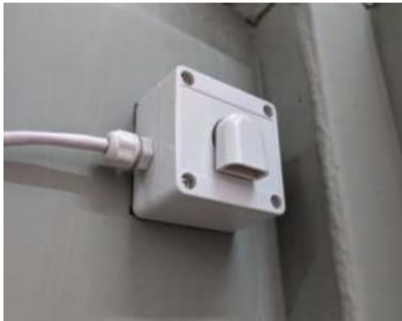
Figure 5: External sensor installed on the transformer.
