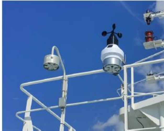
Figure 8: EFOS System installed alongside a commercial EFM system
