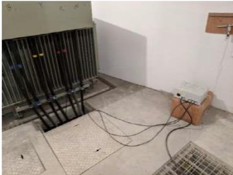
Figure 4: STM device installed at the pilot location
