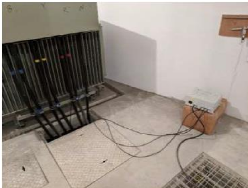
Figure 4: STM device installed at the pilot location
