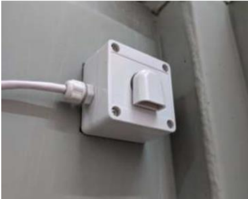
Figure 5: External sensor installed on the transformer.
